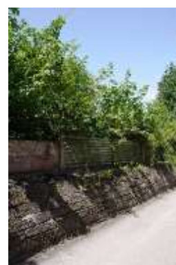
The disused bowling green boundary treatments are in a poor condition
