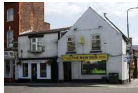
Shops on the Old Market Place in a poor condition, with inappropriate signage, modern windows and painted brickwork.
