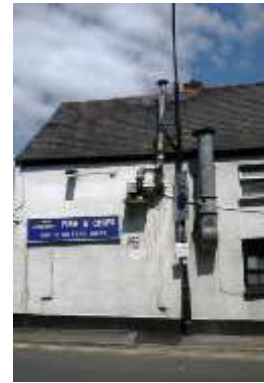
Intrusive ducting and, ventilation inappropriate render in a poor condition and modern signage
